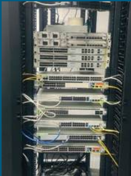
Laboratorio de Networking (Switches y Access Points)
